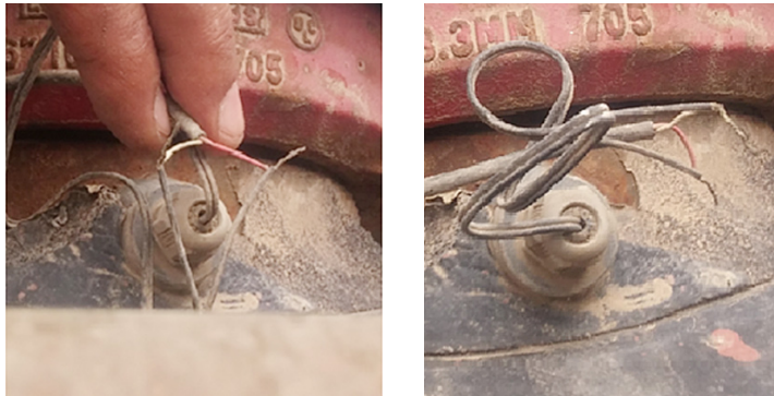
Fig. 4: Sensor wire before repaired
